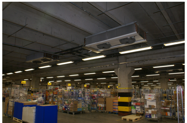
Keslog KV2 central storehouse in Hakkila, Vantaa, a 2009-2010 built machine room, 6 x 500 kW Grasso NH 3 chillers plus air coolers for the dispatch area.
