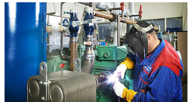
Refrigeration engineering is completed at our plant in Kokkola. We can also carry out 1:1 capacity tests at our testing facility.
