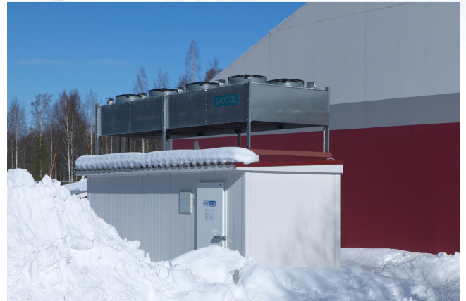
An insulated refrigeration machinery container.(6,8 x 2,5m H=2,4m)
