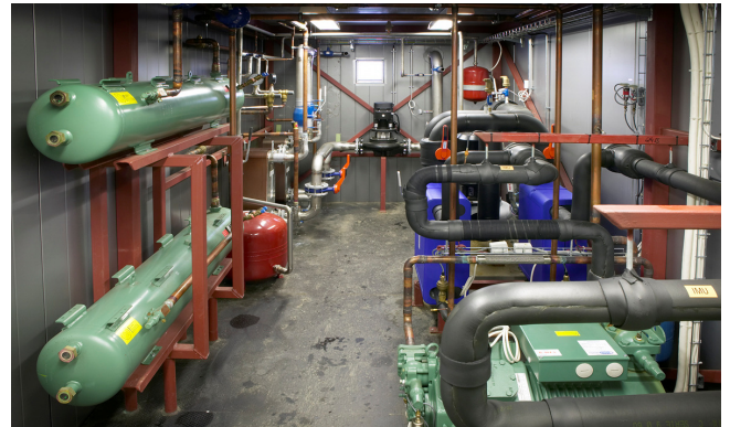
The refrigeration machine room from the inside.
